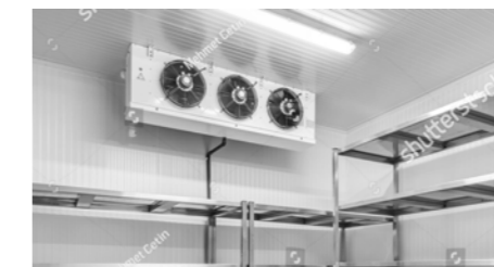
Blaze Freezer Room -35°C
