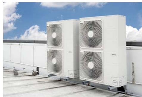
A/C and Refrigeration System
