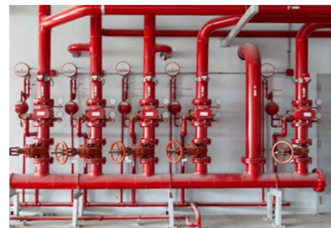
Fire Sprinkler System
