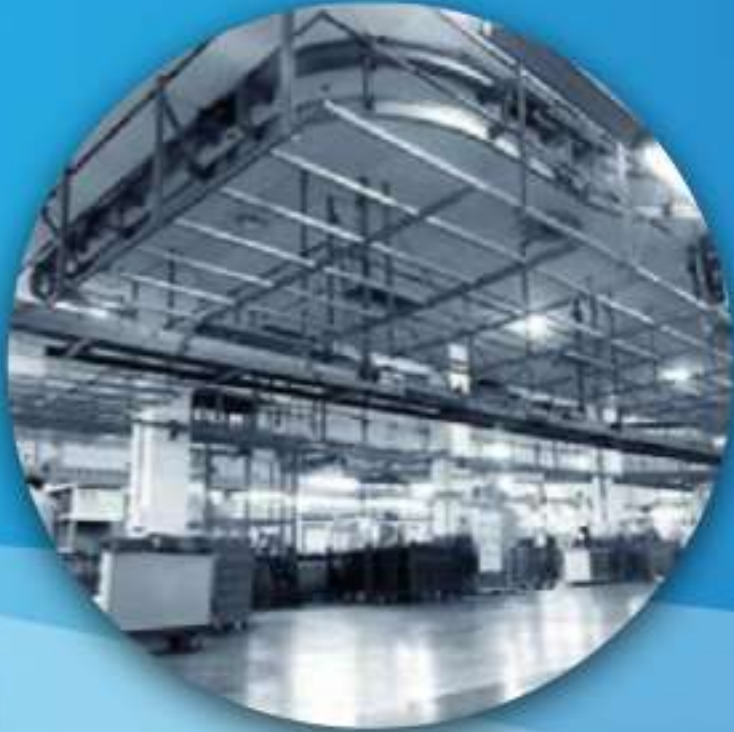
Design and Installation of waterworks, fire safety and HVACR systems
