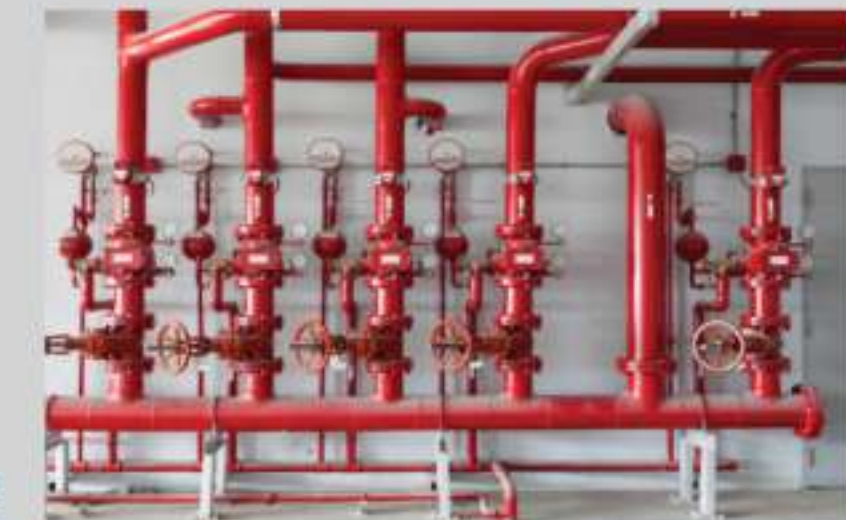
Fire Sprinkler System
